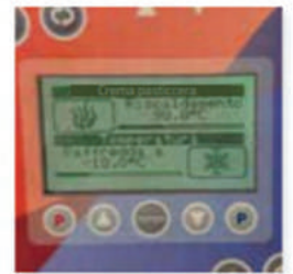
UPPER TANK AND LOWER CYLINDER DIGITAL CONTROL SCREEN
